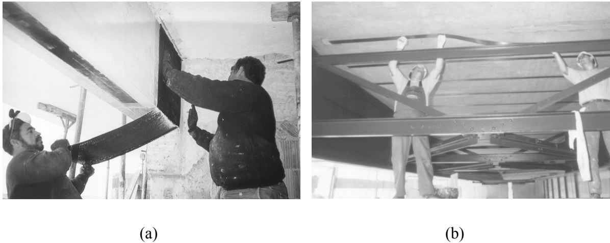
Fig. 2-2: (a) Hand lay-up of CFRP sheets or fabrics. (b) Application of prefabricated strips.
